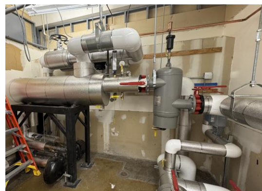
Steam to Hot Water Heat Exchanger (in Room Above)
