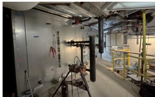
New Single Air Handling Unit
