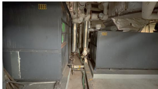
Previous Two Air Handling Units (prior to removal)
