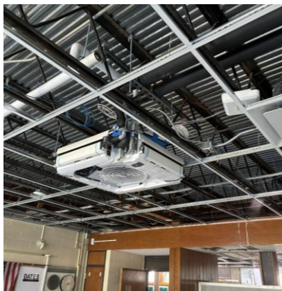
Ceiling-mounted VRF cassette unit providing efficient heating and cooling for classrooms
