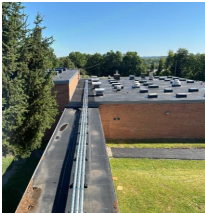
New Rooftop electrical conduits serving the new VRF and ERV systems
